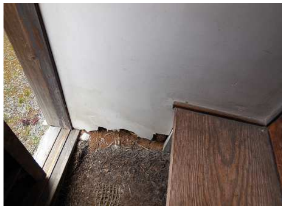
漆喰壁の破損
